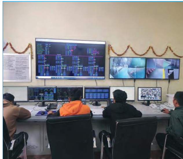
Power House Control Room
