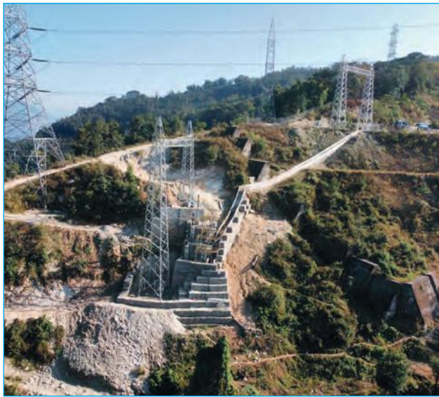
Dhungesanghu Tower to Tower Connection
