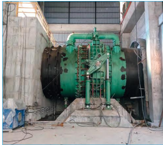
Penstock Protection Valve
