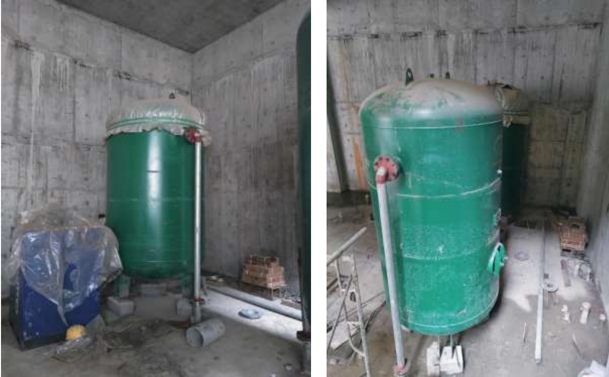
Figure 52: A view of air compressor room
