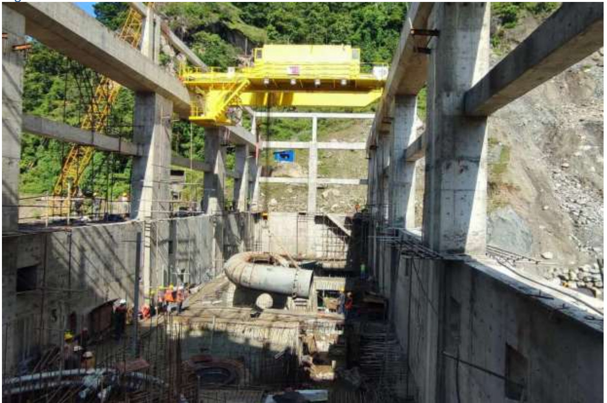
Figure 55: EOT crane being commissioned with the medium load
