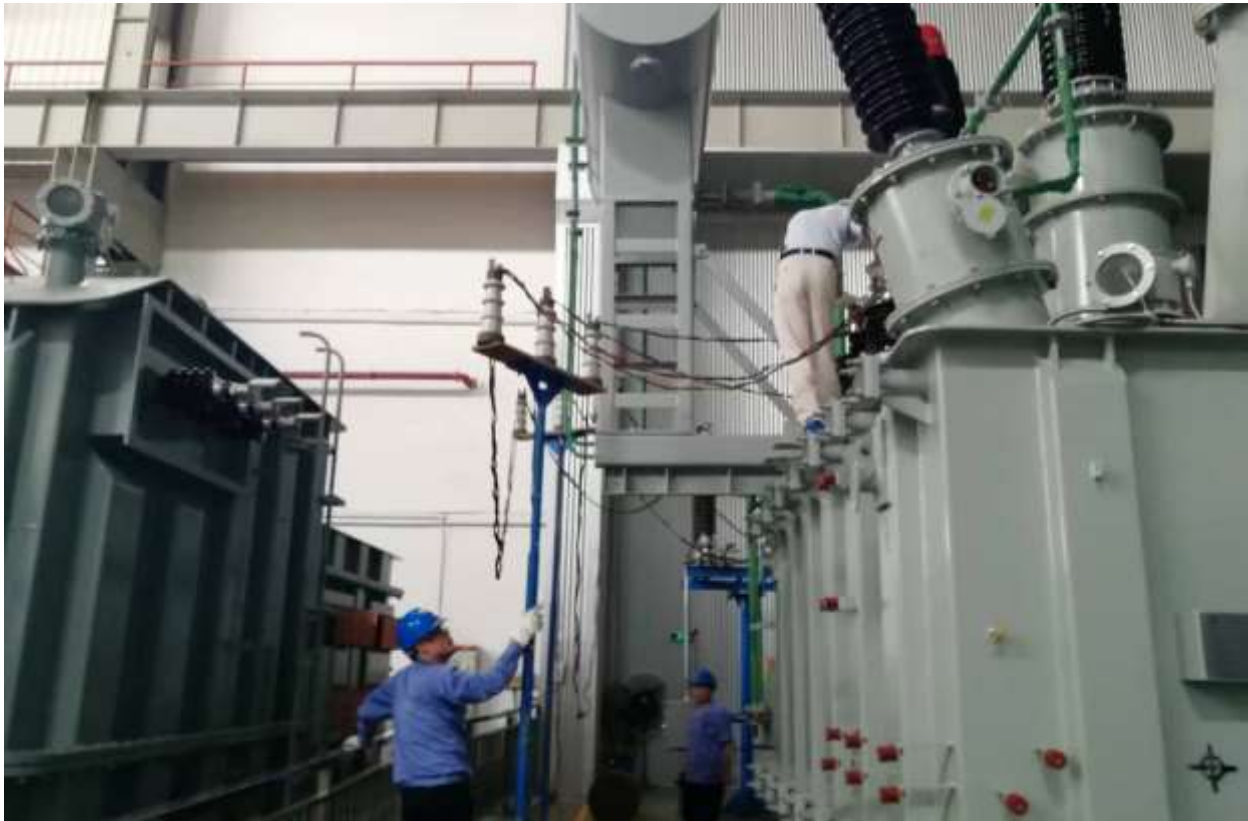
Figure 44: Transformer being factory tested(Contractor's factory in China)
