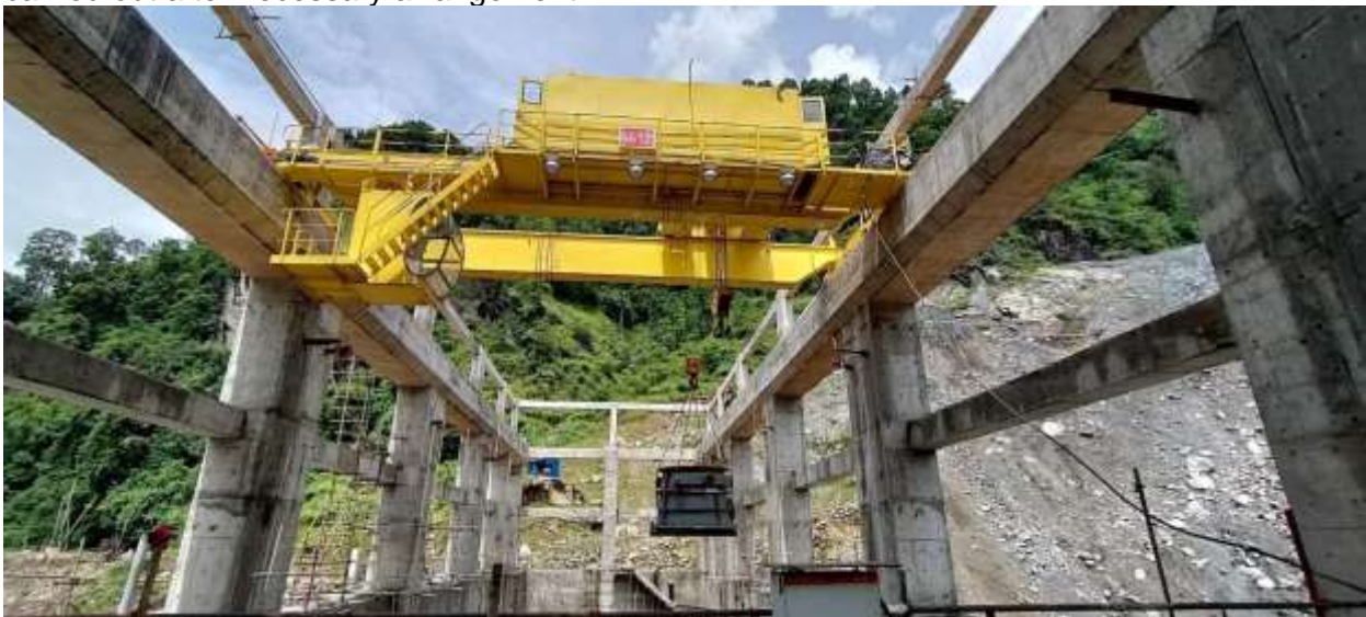
Figure 53: EOT crane being commissioned with small load
