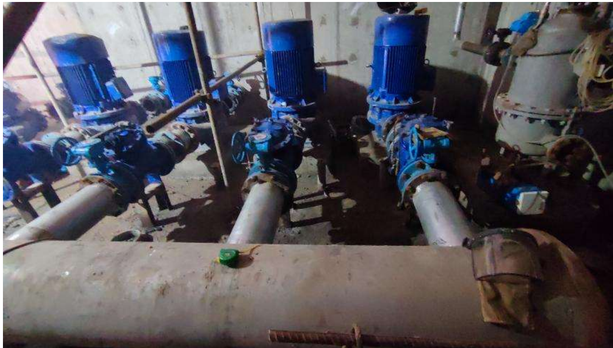
Figure 51: A view of water cooling pumps and the filter
