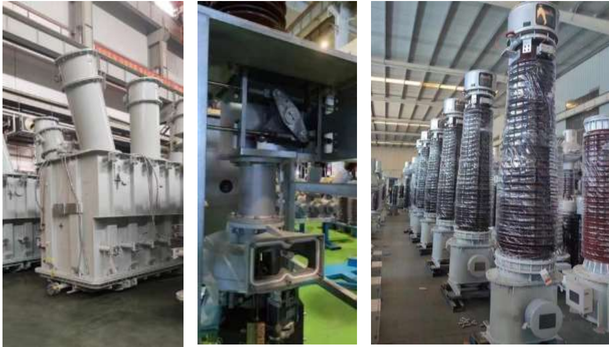
Figure 46: A view of Transformer and switchgear (Contractor's factory in China)
