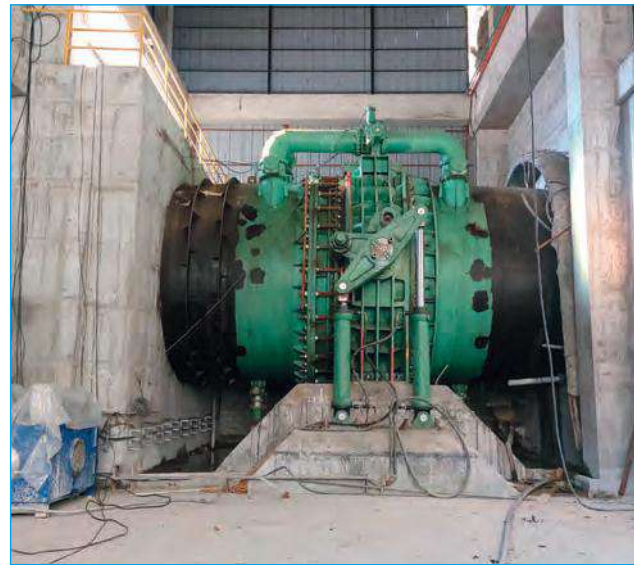
Penstock Protection Valve
