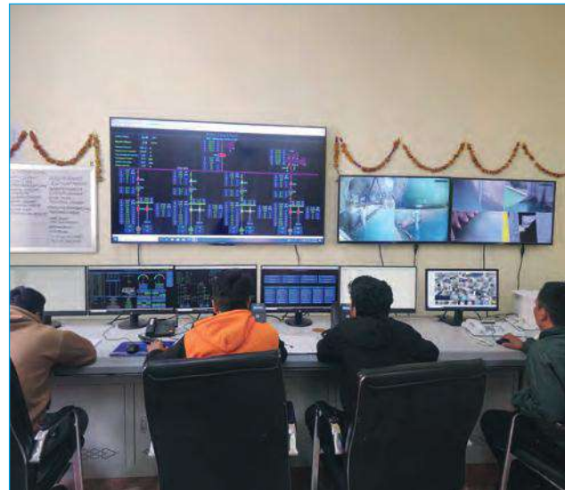
Power House Control Room
