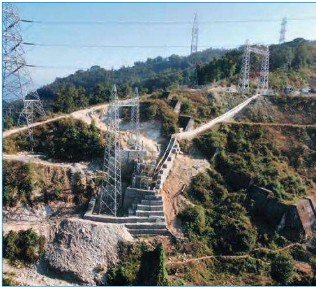
Dhungesanghu Tower to Tower Connection
