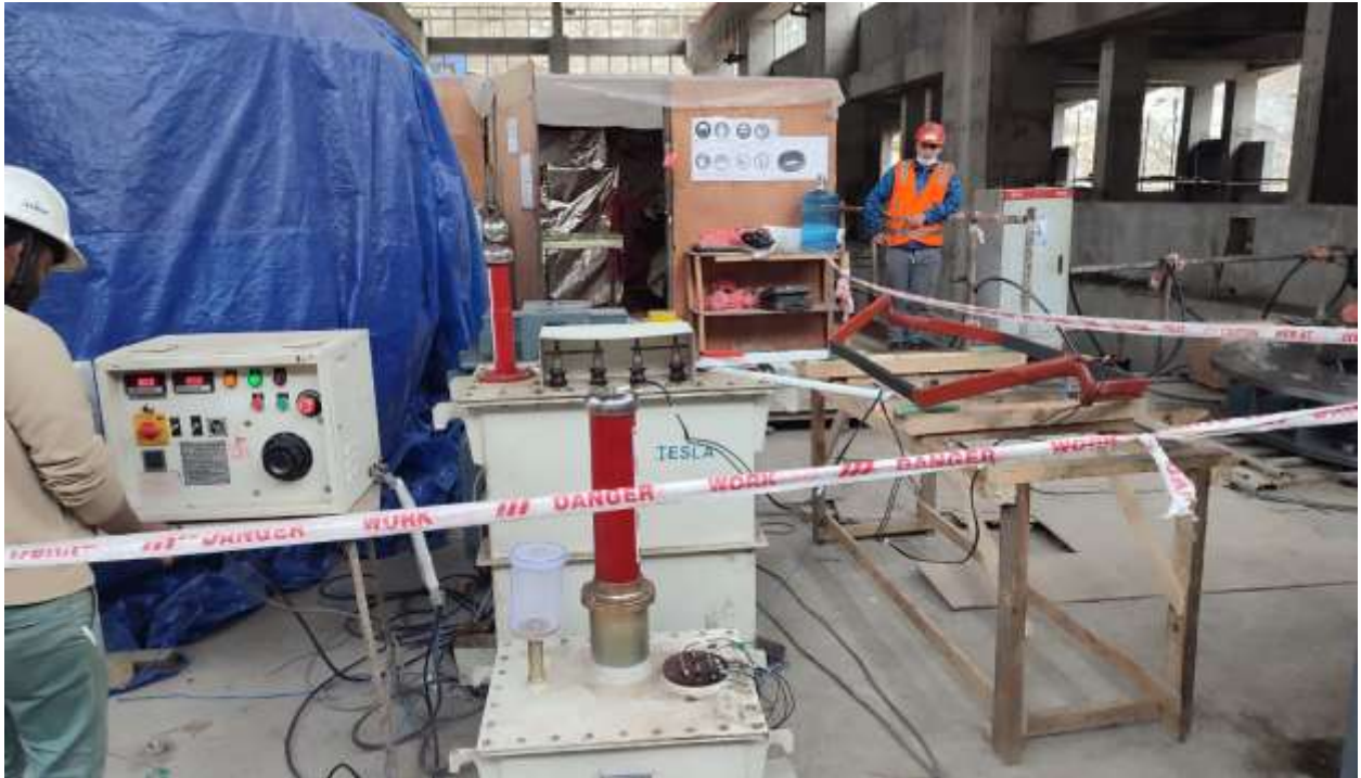
Figure 54: High voltage test of stator coil
