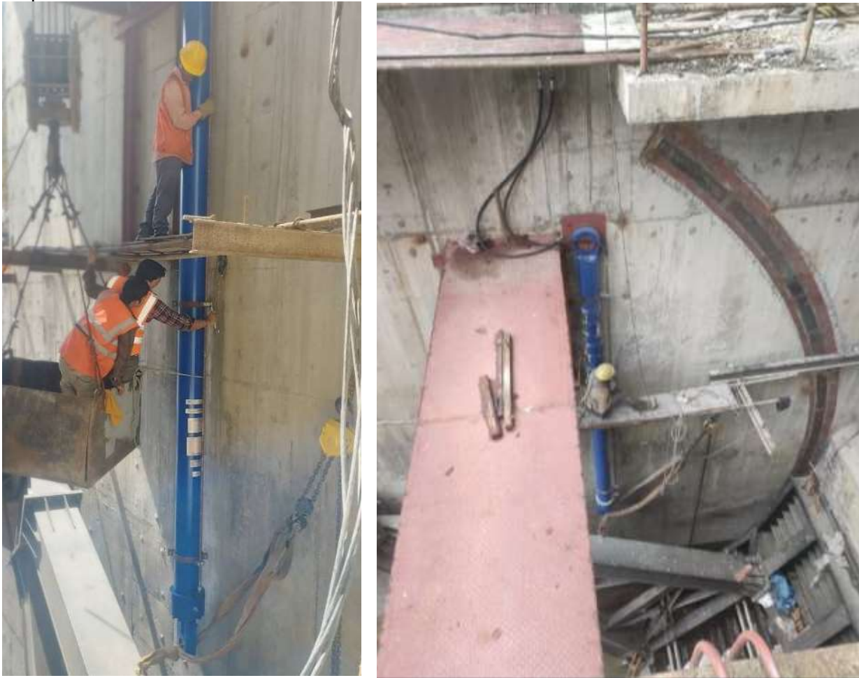
Figure 2-31: Erection of hydraulic hoisting cylinders of radial gate (left) and hydraulic arm of radial gate of intake side (right)
