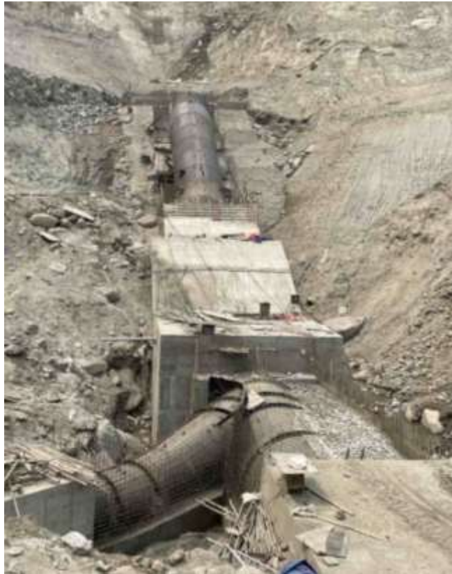
Figure 2-28: A view of erection of penstock pipes and bifurcation unit 01 during installation
