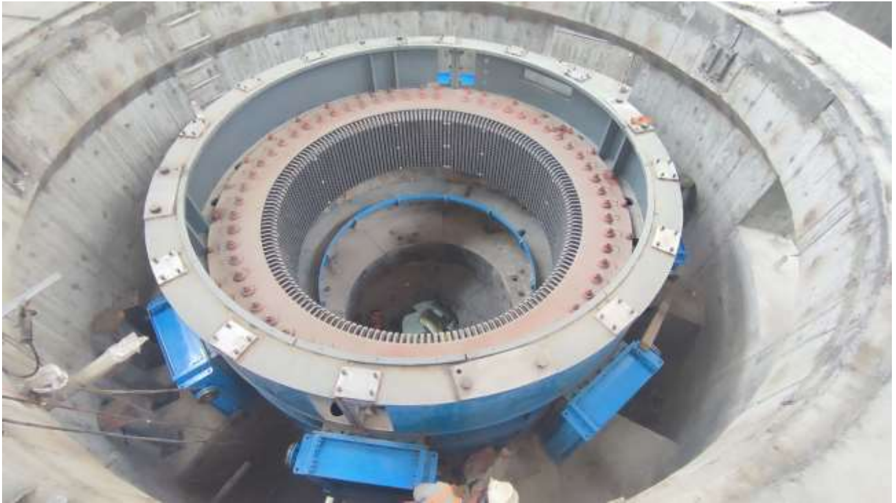
Figure 65: Stator air cooler assembly
