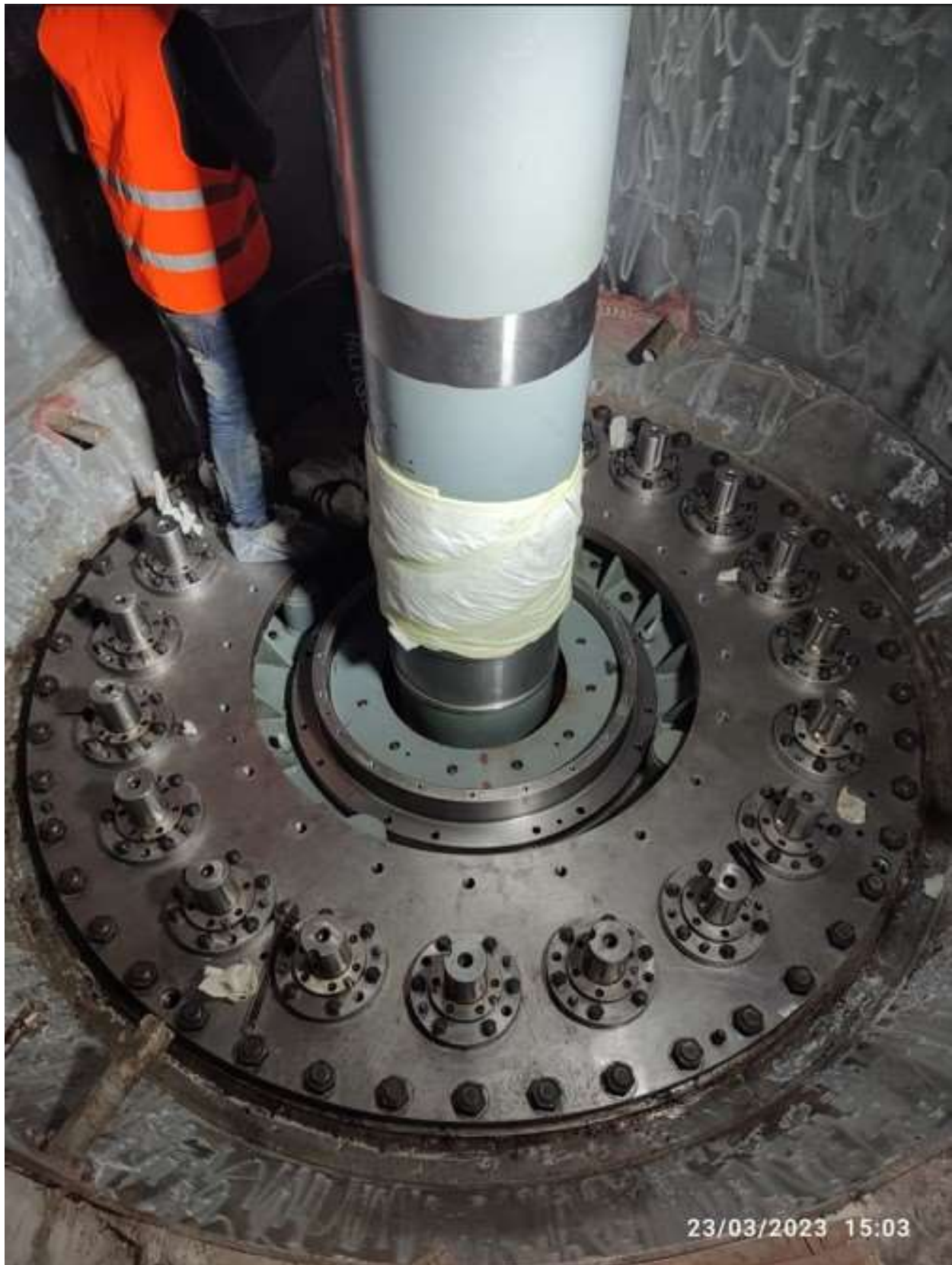
Figure 2-44: Final assembly of bottom ring, guide vane, head cover and main shaft with runner
