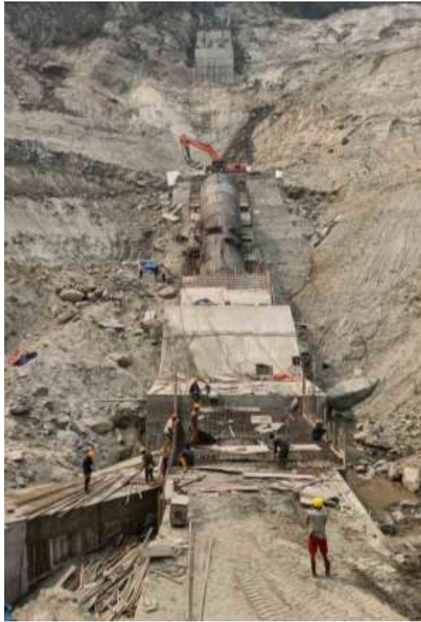
Figure 2-22: A view of concreting works and pipe erection works along penstock alignment
