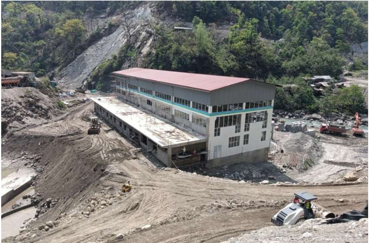
Figure 2-20: A view of powerhouse and manifold
