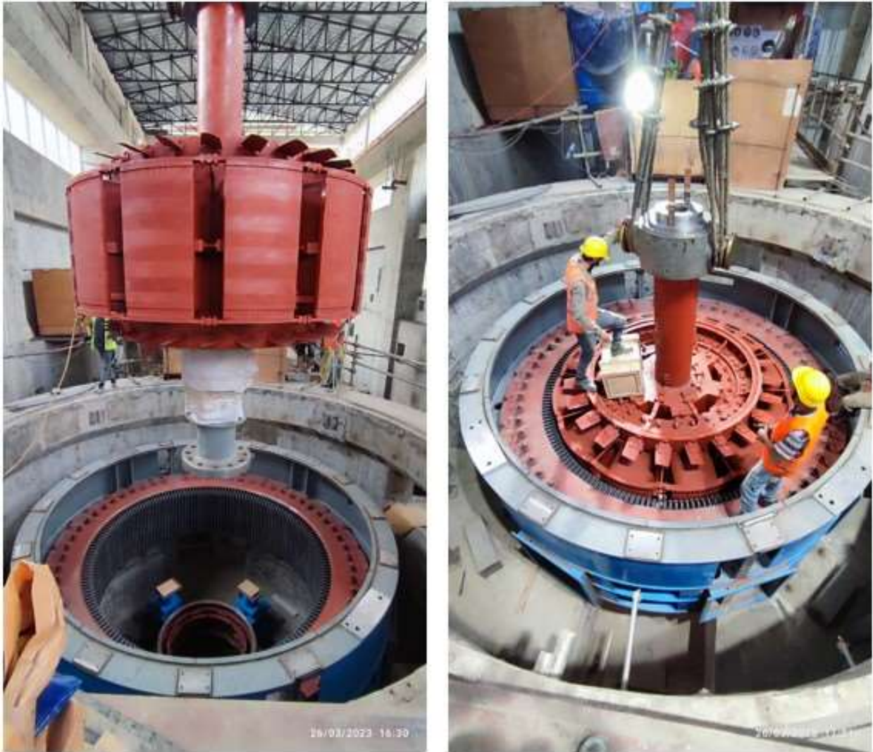
Figure 2-47: Temporary parking of rotor of unit 01 at unit 02
