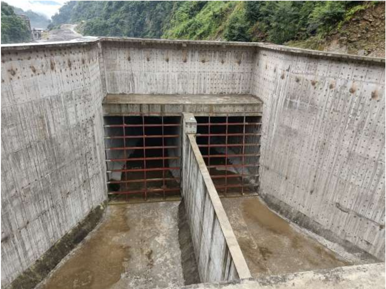
Figure 2-8: A view of conveyance tank
