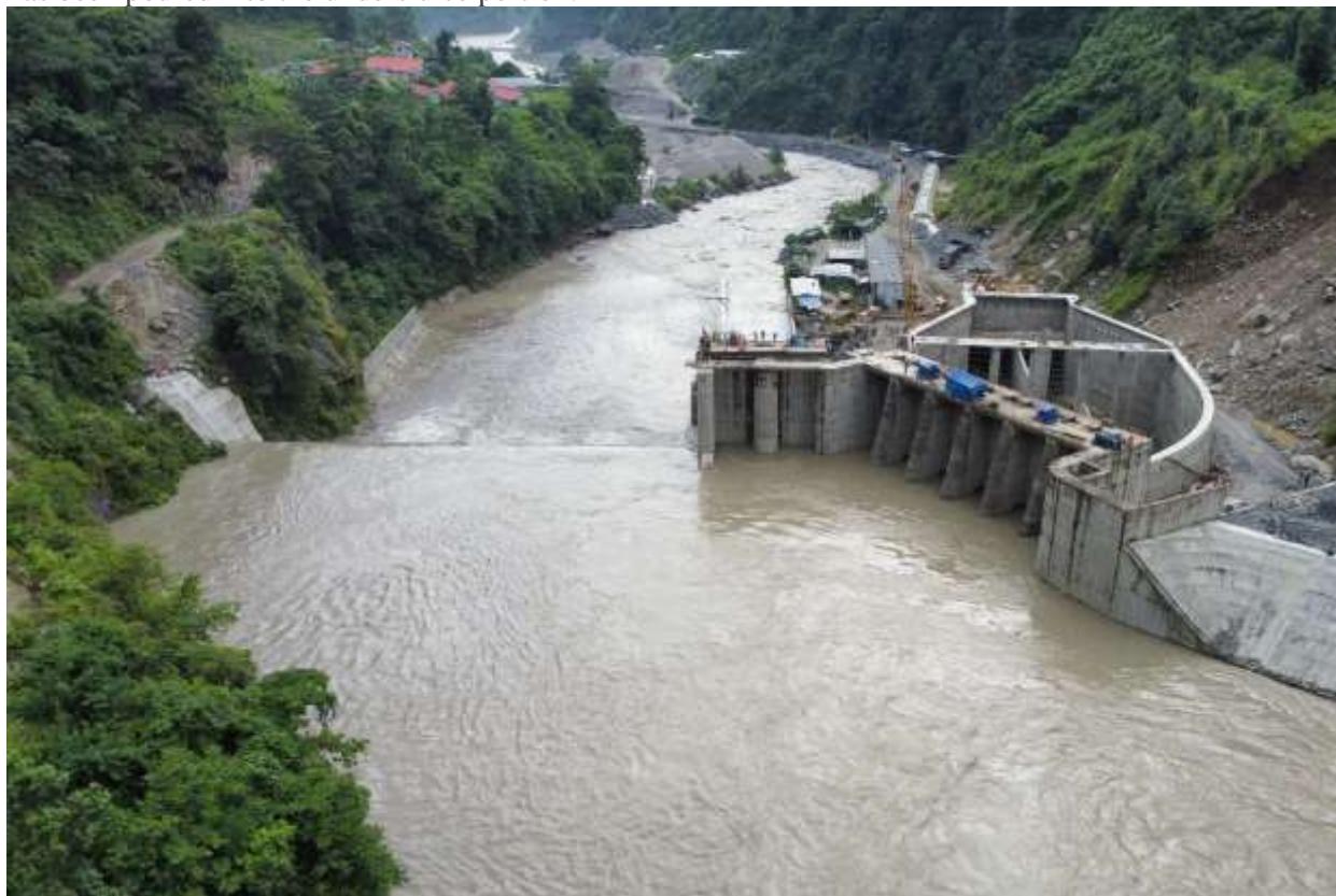
Figure 2-7: A view of headworks during water filling test
