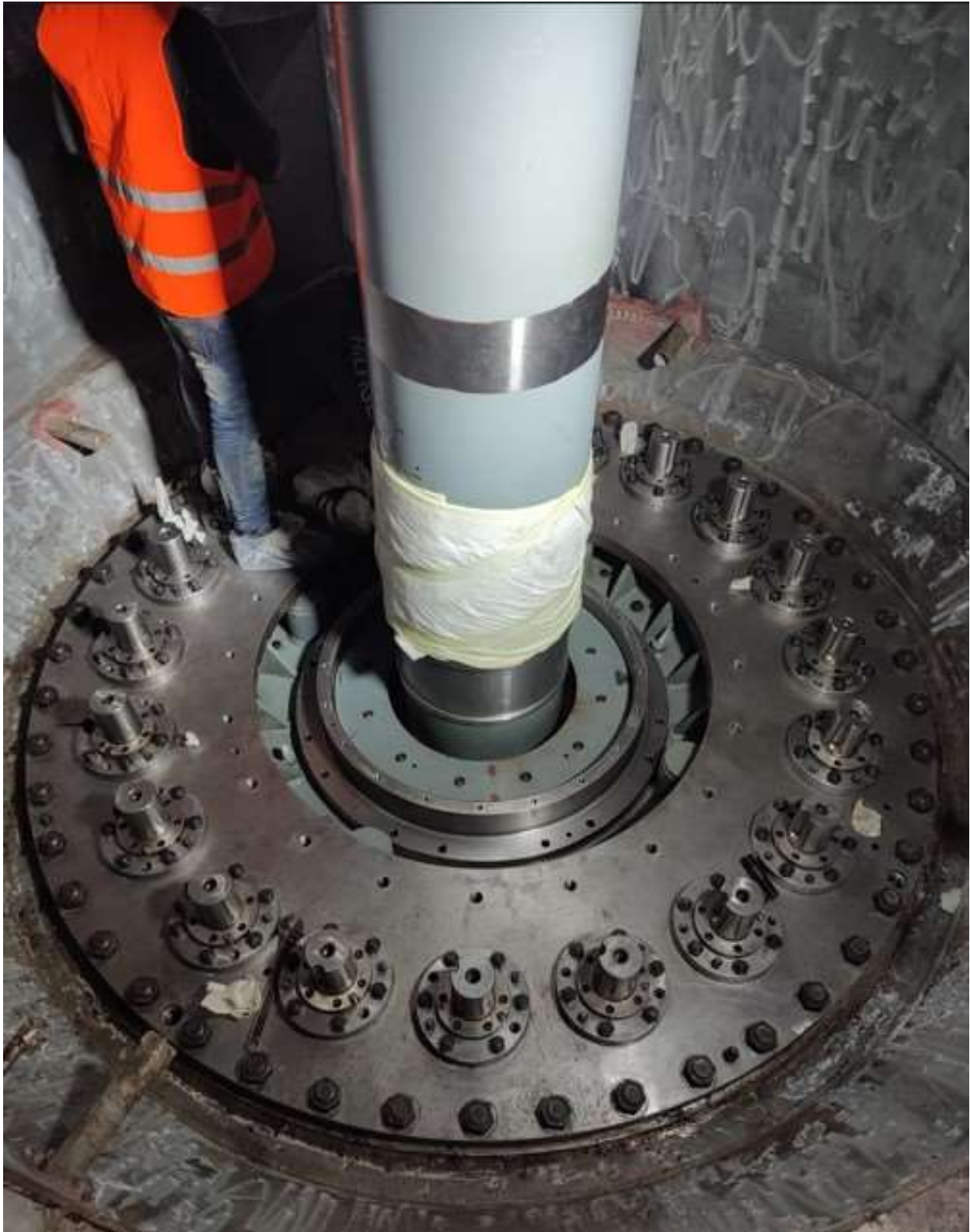
Figure 2-64: Final assembly of bottom ring, guide vane, head cover and main shaft with runner
