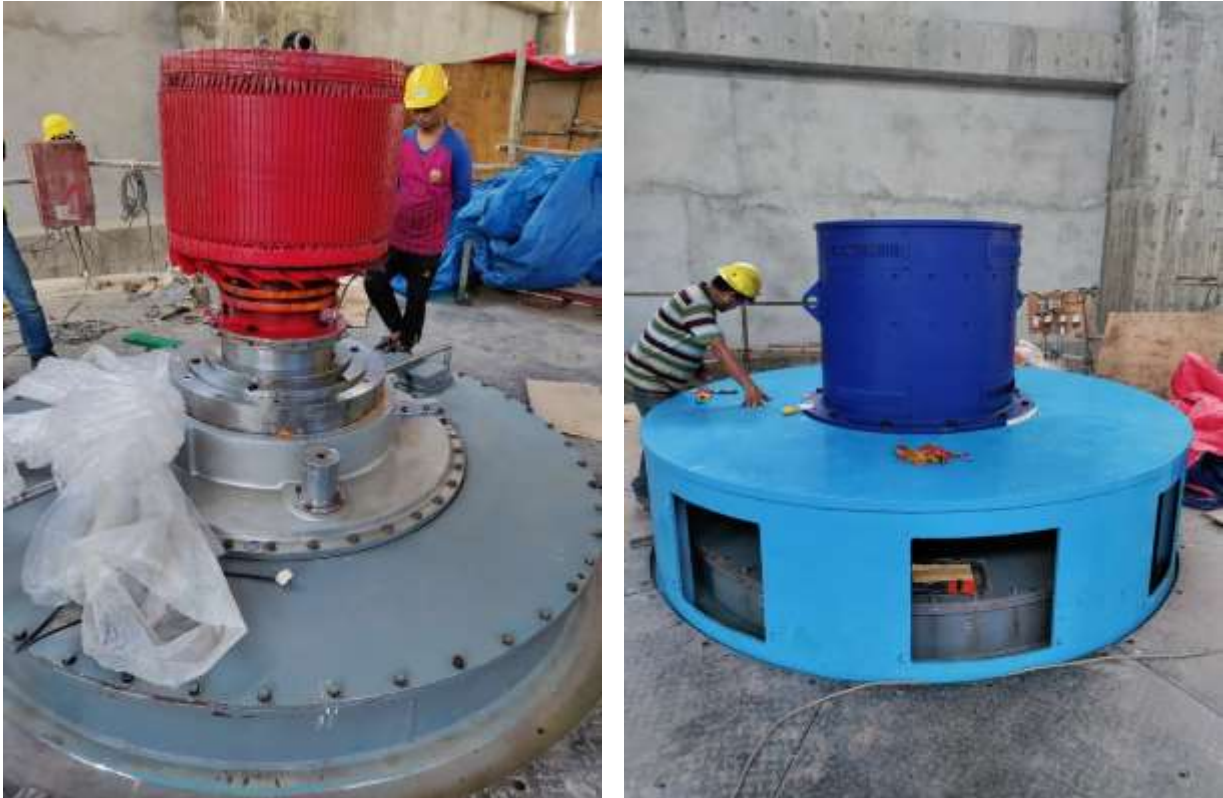
Figure 2-57: Pressure test of upper bracket bearings oil cooler
