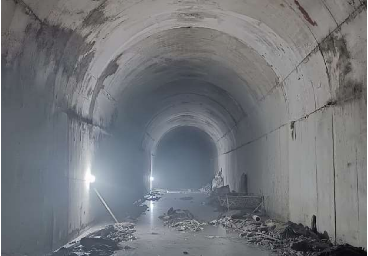
Figure 2-19: A section of HRT with concrete full lining from the adit region
