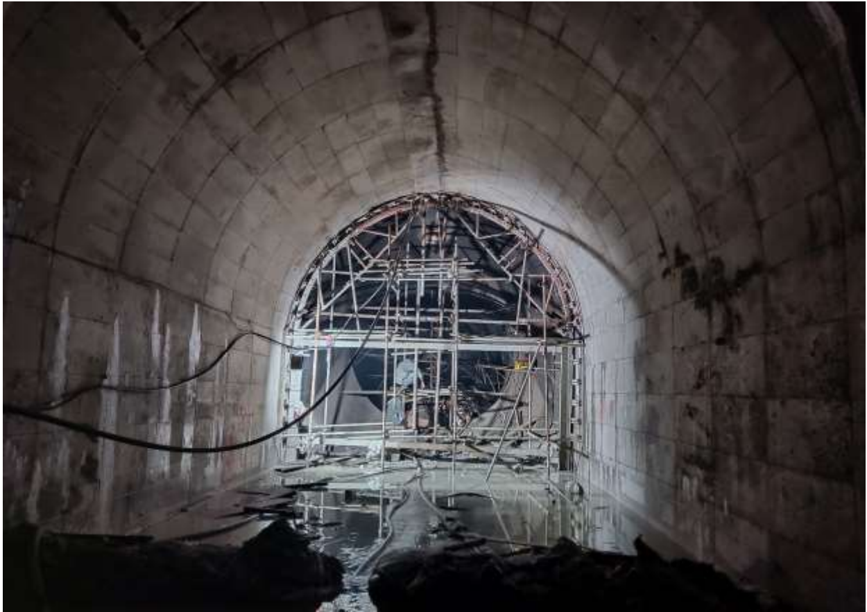
Figure 2-21: A section of HRT with concrete full lining from the outlet region
