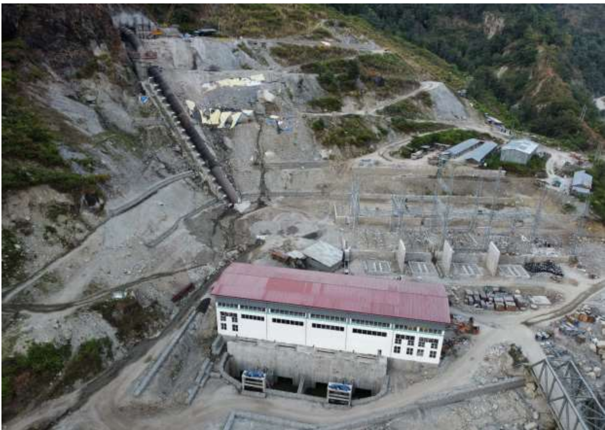
Figure 2-30: A view of the construction works of transformer foundation at switchyard region
