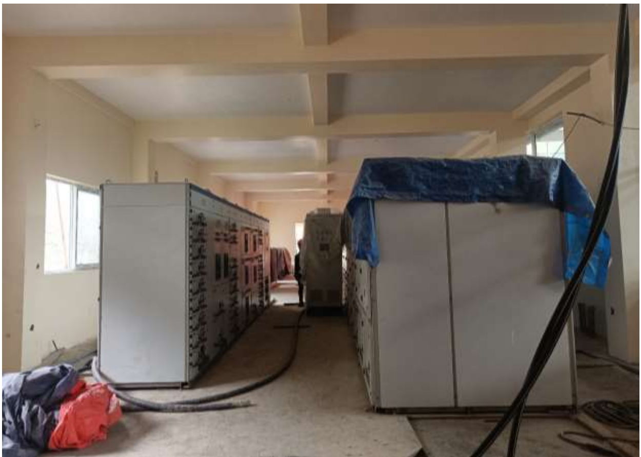
Figure 2-36: Interior view of powerhouse auxiliary building (control bay)
