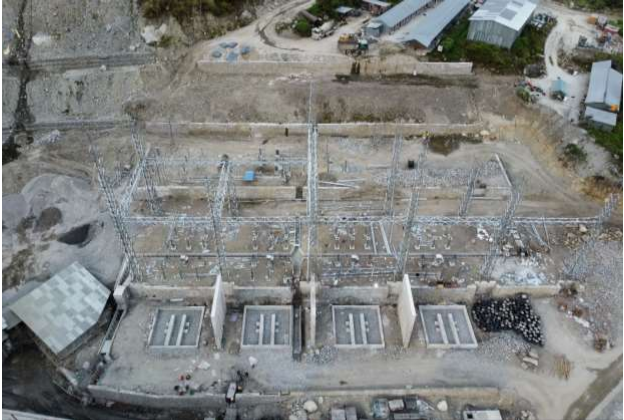
Figure 2-31: A view of switchyard
