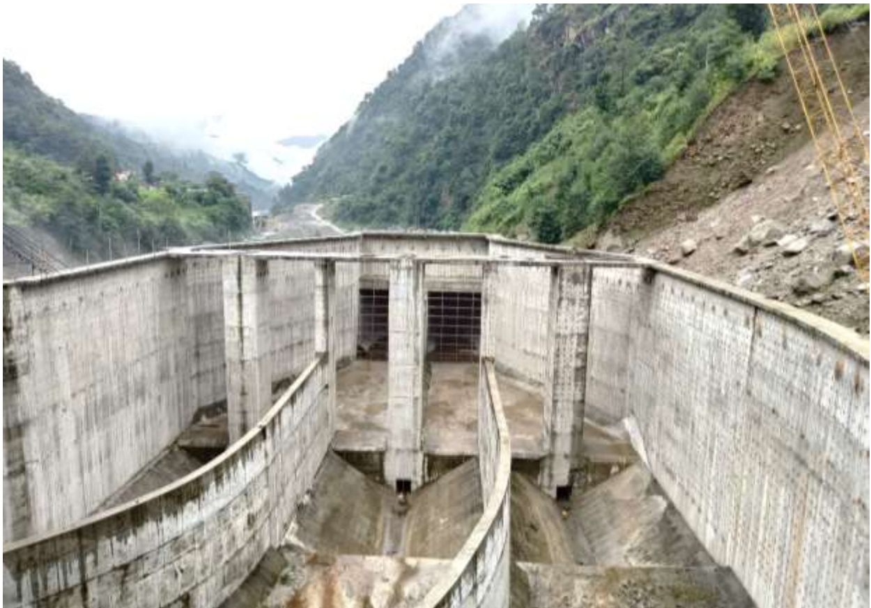
Figure 2-5: A view of gravel trap and conveyance tank from upstream
