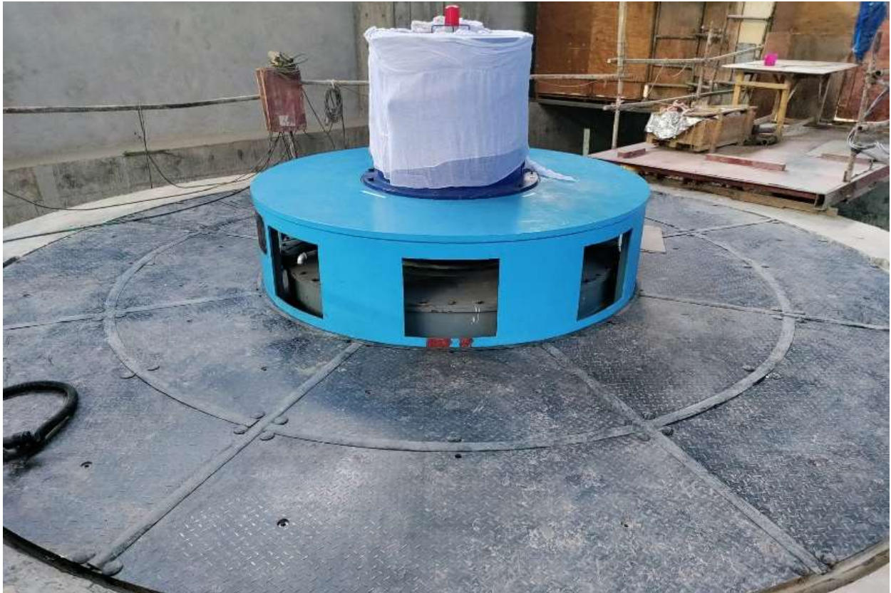
Figure 54: Final installation of excitation system
