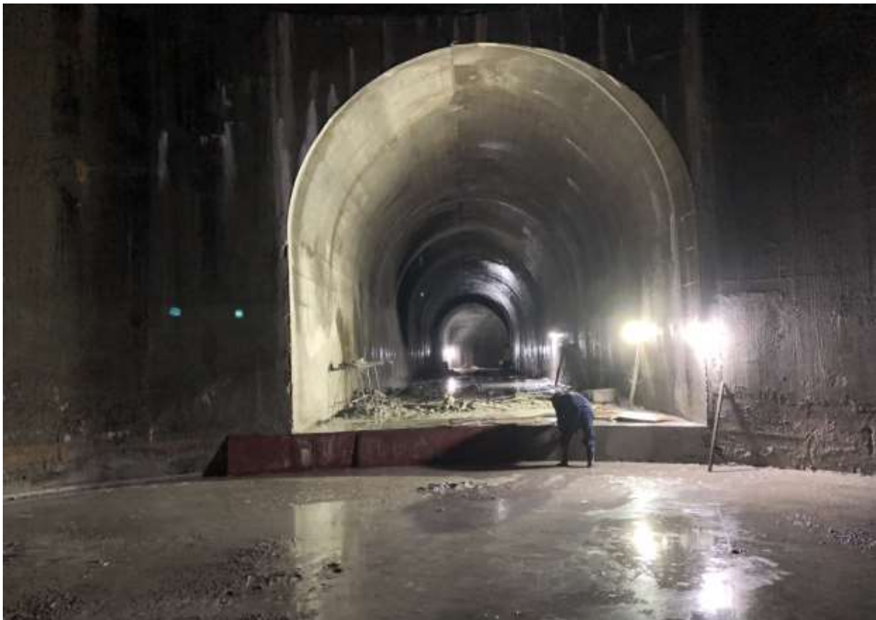
Figure 2-27: A view of full lining concrete at connecting tunnel of Surge Shaft
