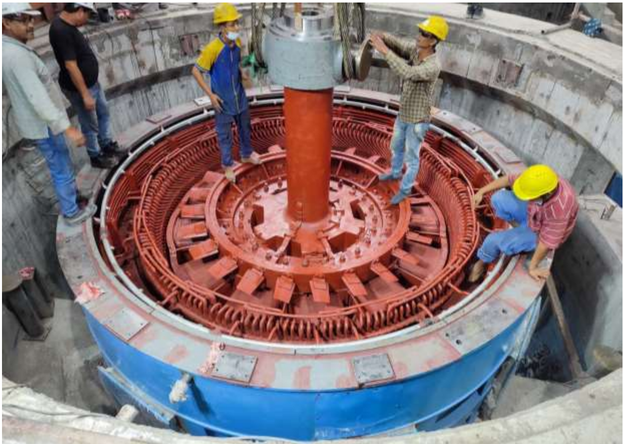
Figure 2-52: Rotor and stator coupling in unit 01
