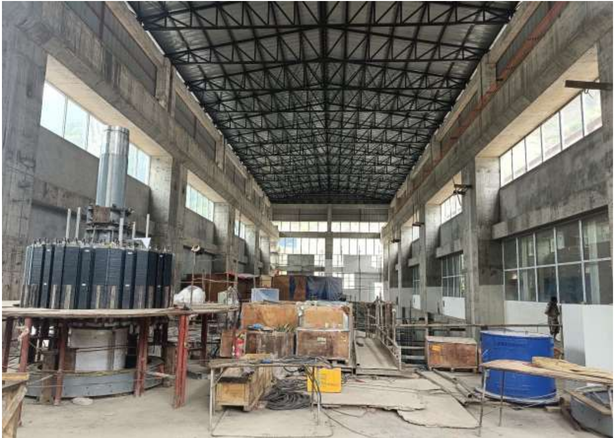
Figure 2-35: Interior view of powerhouse main building
