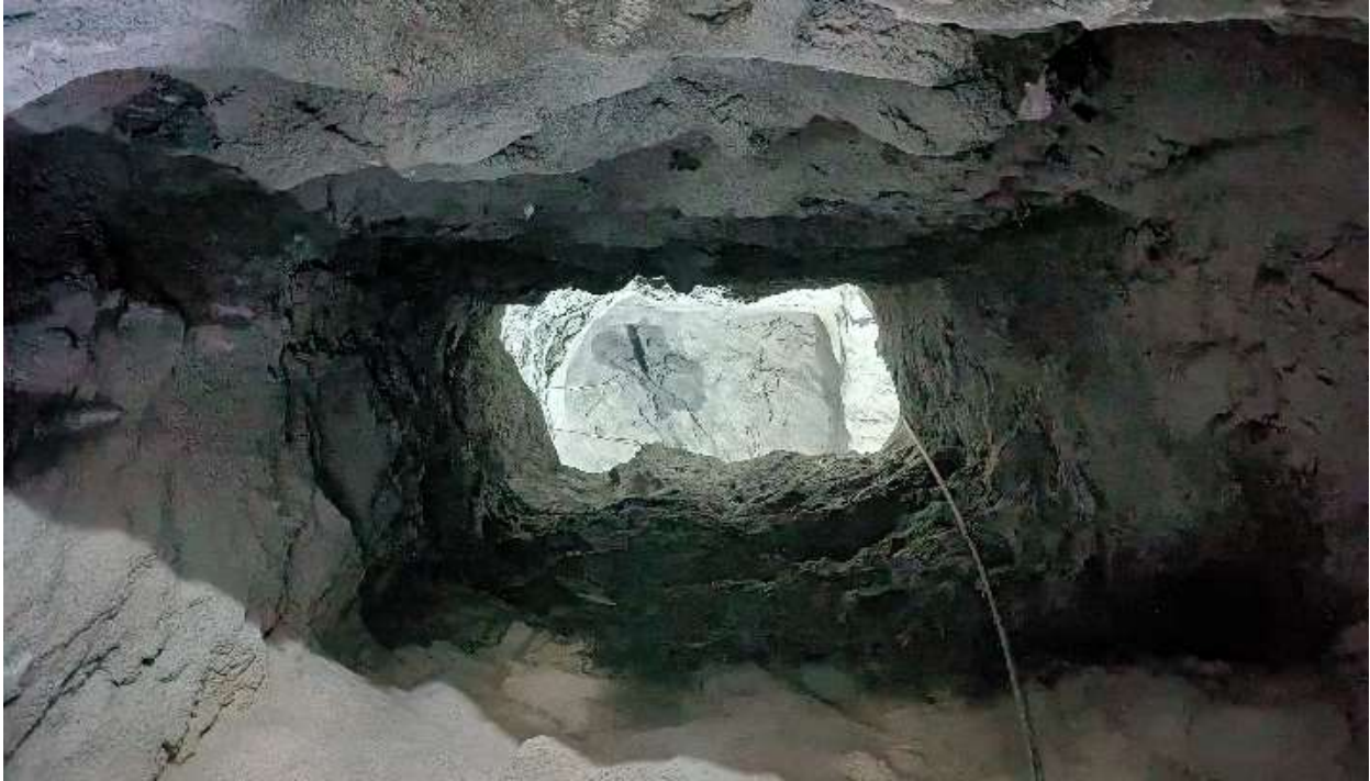
Figure 2-23: A view of settling basin inlet gate 03 (top view from inspection tunnel 01)
