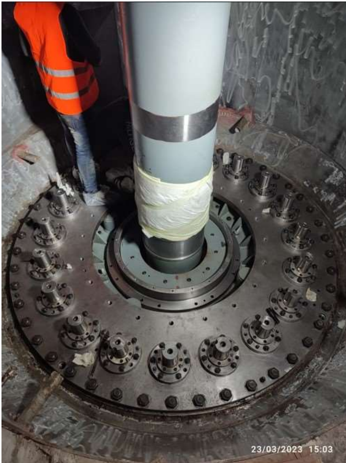
Figure 2-60: Final assembly of bottom ring, guide vane, head cover and main shaft with runner
