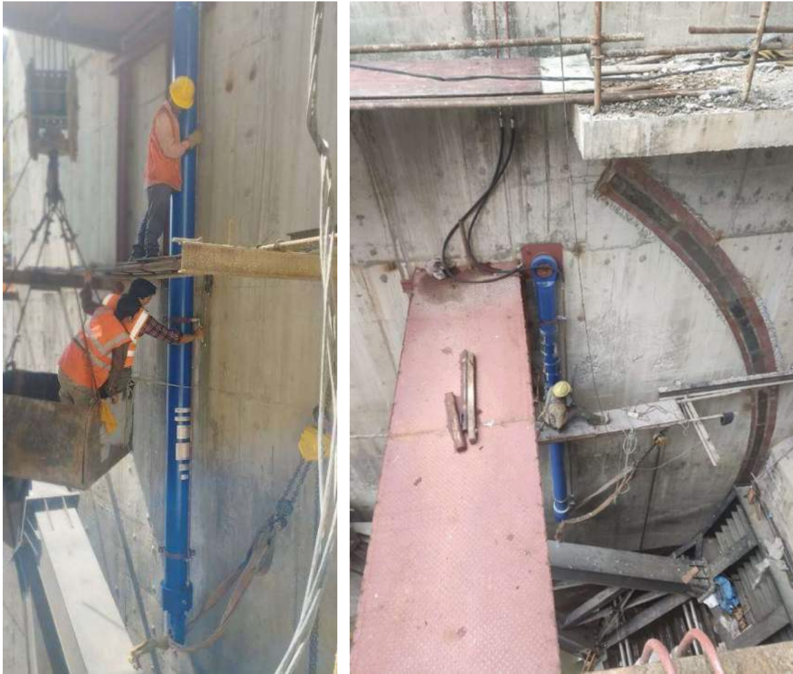
Figure 2-43: Erection of hydraulic hoisting cylinders of radial gate (left) and hydraulic arm of radial gate of intake side (right)
