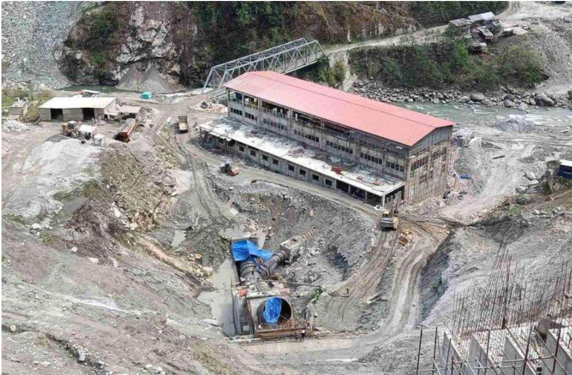
Figure 2-24: A view of powerhouse and manifold from outlet portal region
