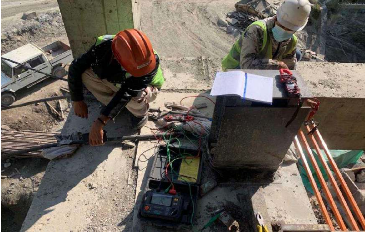
Figure 2-54: Insulation Resistance of EOT's busbar
