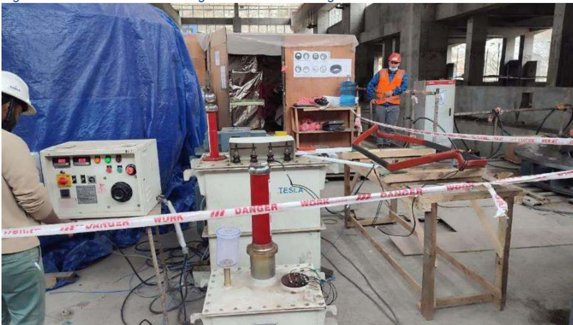
Figure 2-57: High voltage test of stator coil
