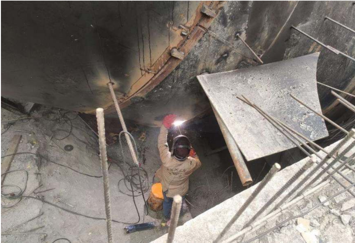
Figure 2-37: Welding work at pipe of dia 4.5 m and thk 32 mm from outside
