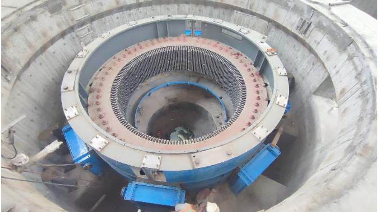
Figure 65: Stator air cooler assembly
