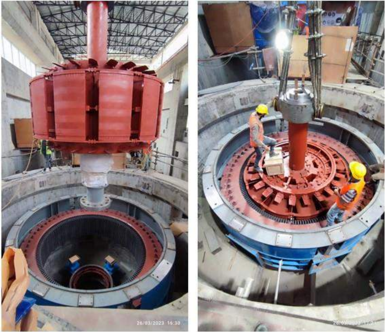
Figure 2-36: Temporary parking of rotor of unit 01 at unit 02
