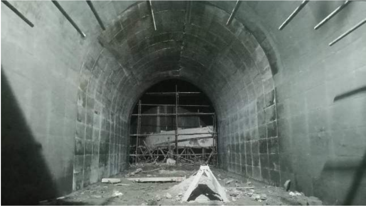
Figure 2-15: A view of full lining concrete at connecting tunnel to Surge Shaft
