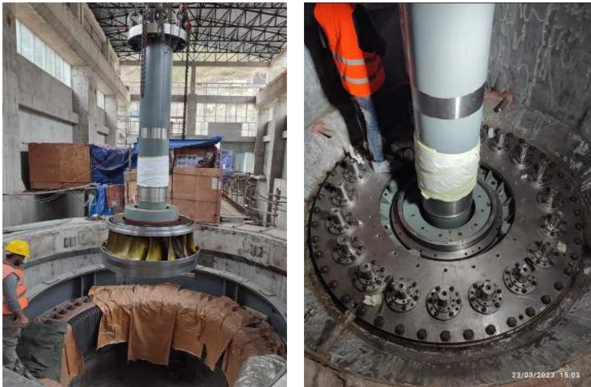
Figure 2-34: Lowering of runner with main shaft in unit 2 (left) and final assembly of bottom ring, guide vane, head cover and main shaft with runner (right)
