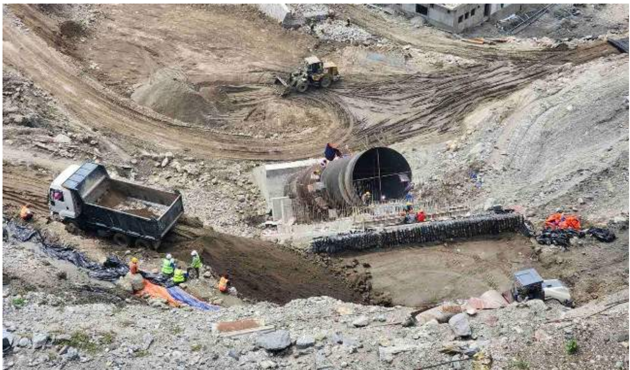
Figure 2-20: A view of concreting works and pipe erection works along penstock alignment
