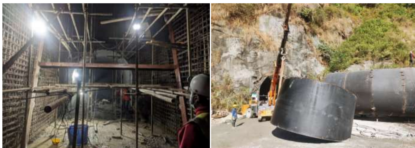
Figure 2-17: Erection of trash rack frame and gate embedded parts at SB Outlet Gate-3 (left) and installation of head race bend (right)
