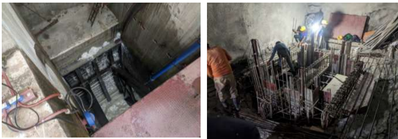
Figure 2-19: Erection of radial gate at undersluice (left) and erection of embedded part of gate and stoplog at SBF-3 (right)
