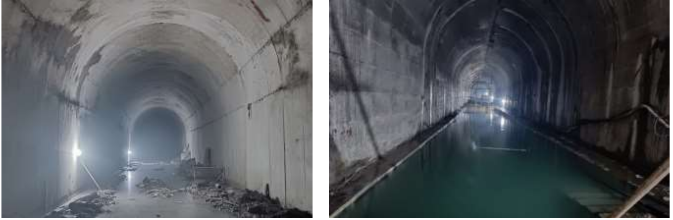
Figure 2-11: A section of HRT with concrete full lining from the adit region (left) and A completed section of rock trap (right)
