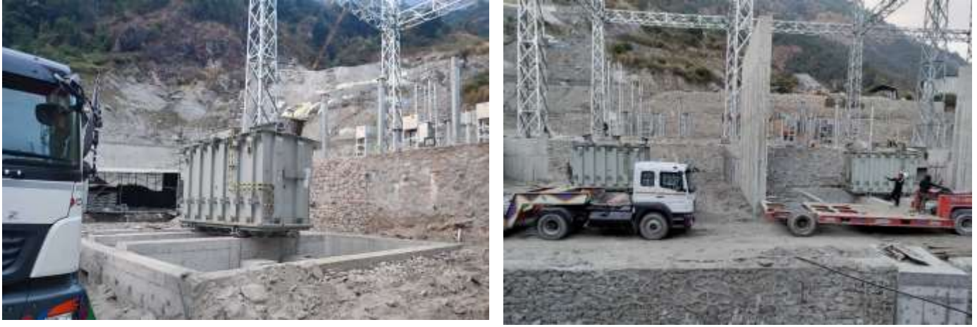
Figure 2-26: Power transformers placed at its position (left) and unloading of power transformers at the switchyard region (right)
