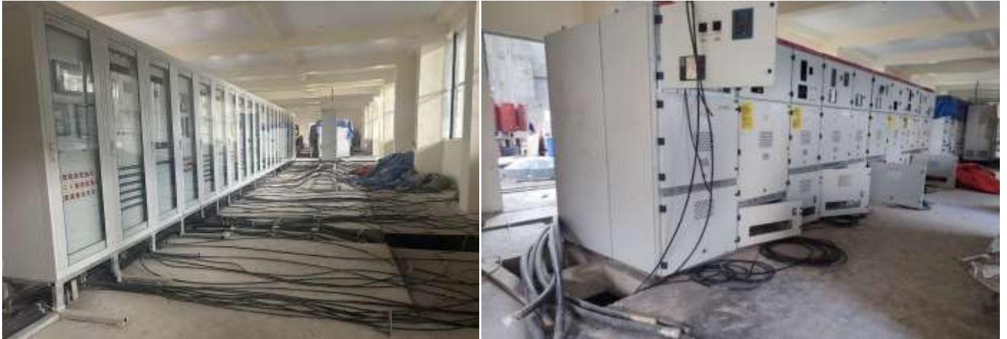
Figure 2-24: Laying of control cables in control room (left) and laying of power and control cables in 11kV switchgear room (right)
