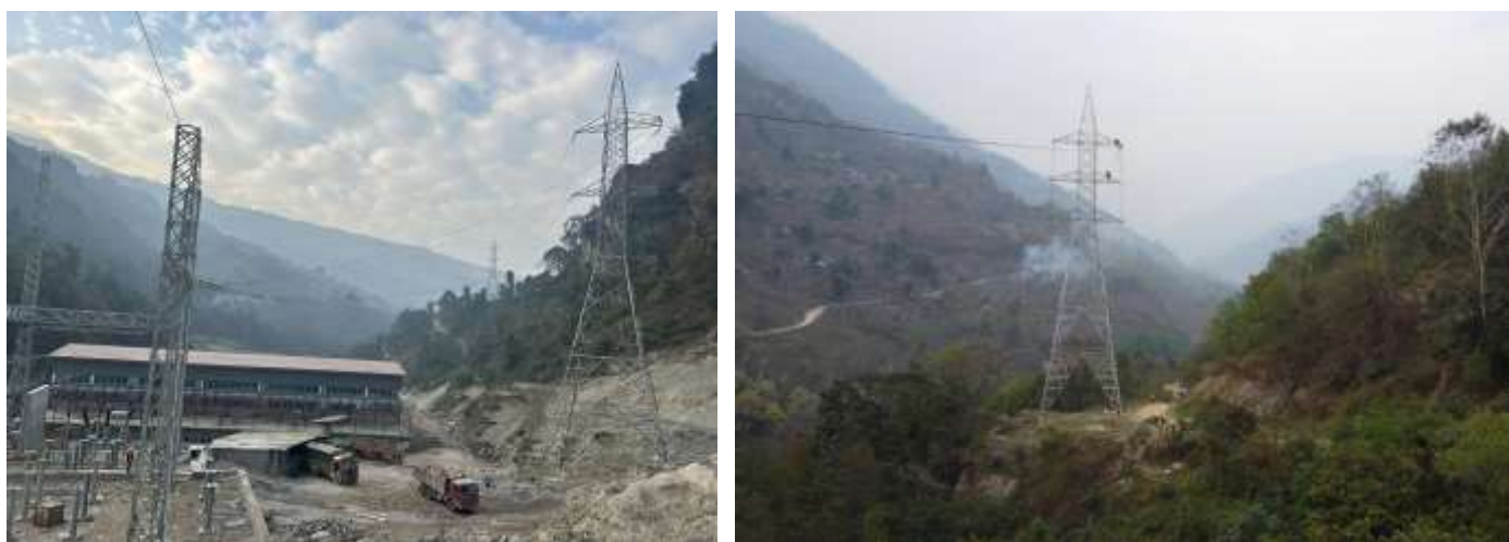
Figure 2-28: View of Conductor stringing from switchyard gantry to AP1 (left) and a view of stringing works (right)
