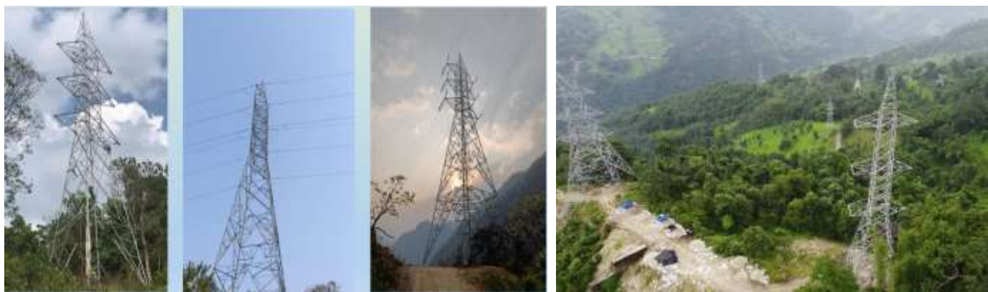
Figure 2-29: Photographs showing stringing works (left) and erected last tower at AP24 and tower of NEA (right)
