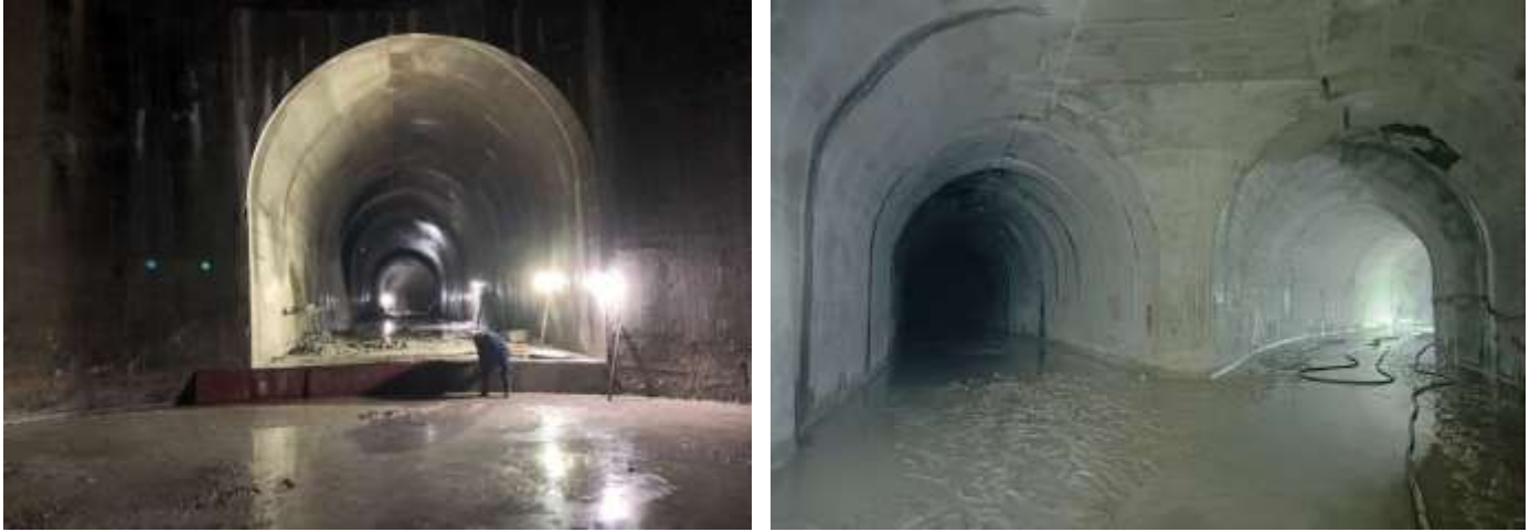
Figure 2-13: A view of full lining concrete at connecting tunnel (left) and the junction of connecting tunnel and HRT (right)
