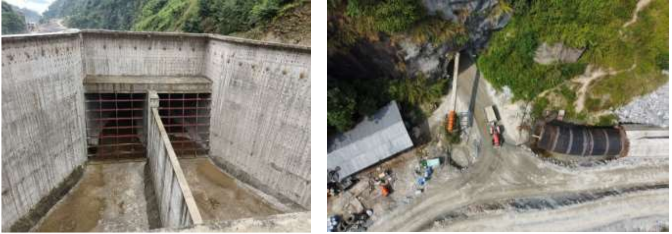
Figure 2-4: A view of conveyance tank (left) and Approach pipes installation completed upto inlet portal (right)
