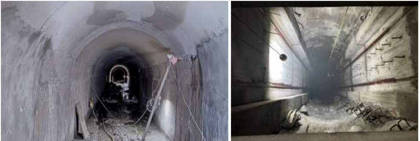
Figure 2-12: A view of full concrete lining at the flushing tunnel (left) and Concreting works at flushing shaft 1'A' (right)
