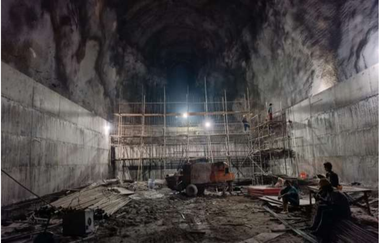
Figure 2-11: A view of concrete lining works being carried out at Settling basin 01
