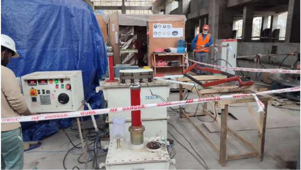
Figure 54: High voltage test of stator coil
