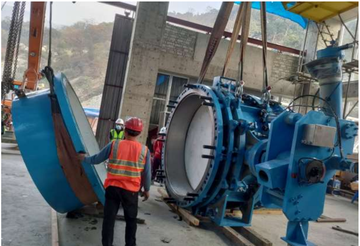
Figure 2-48: Unit 2 MIV assembled at Service bay
