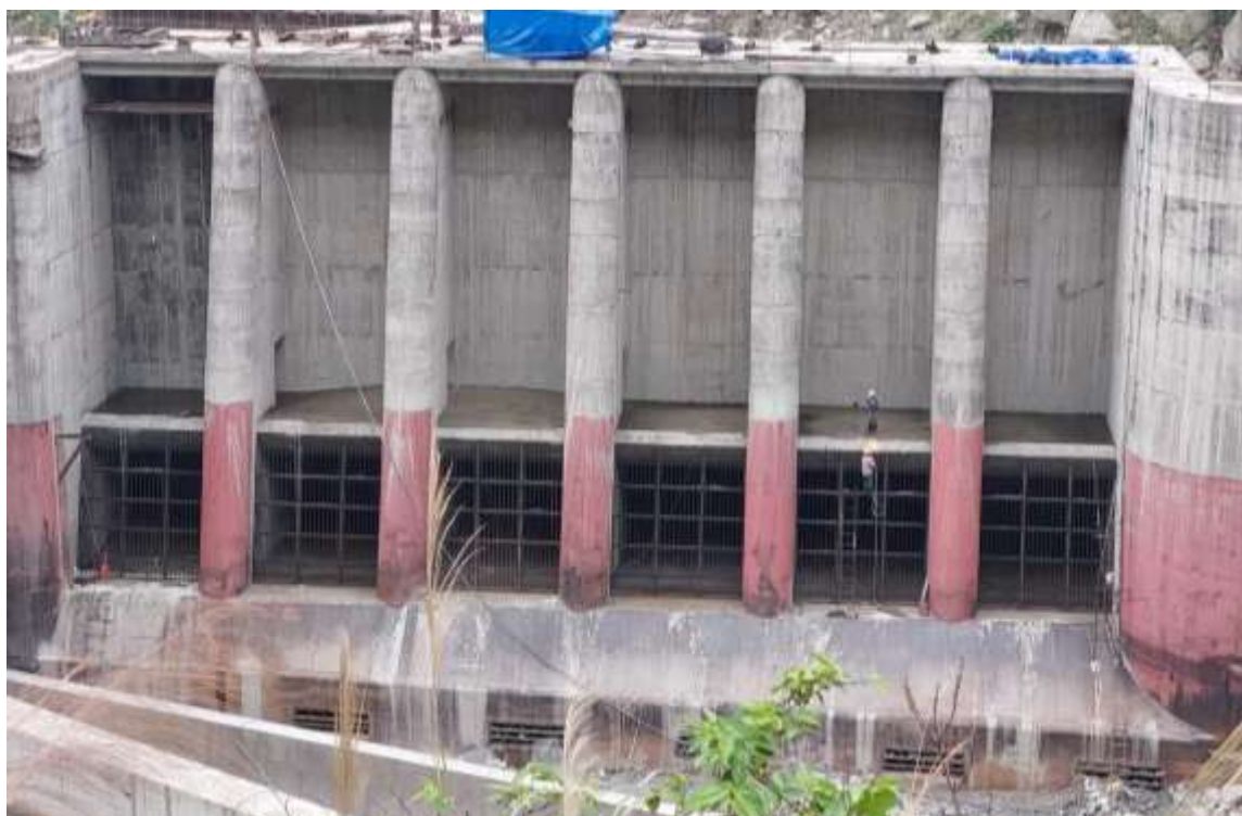
Figure 2-5: A front view of intake orifices
