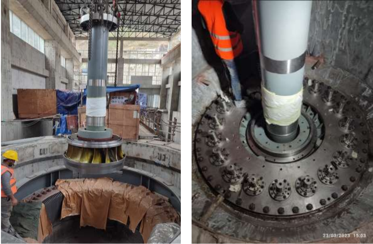
Figure 2-43: Lowering of runner with main shaft in unit 2 (left) and final assembly of bottom ring, guide vane, head cover and main shaft with runner (right)
