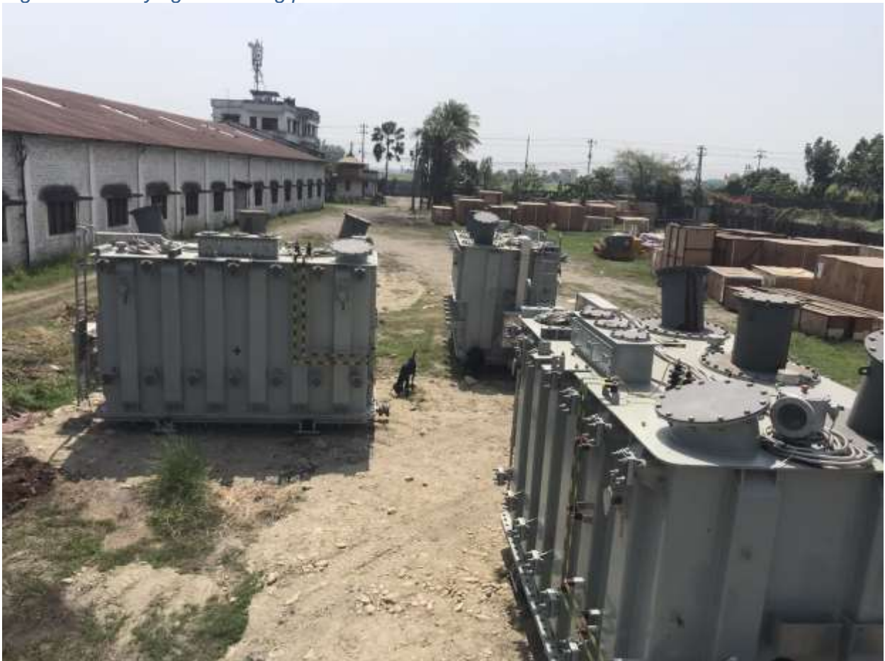
Figure 2-51: Storage of transformers at Biratnagar yard
