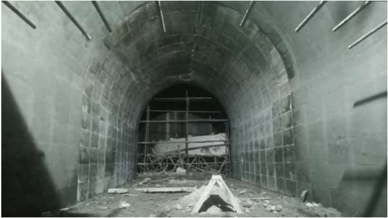
Figure 2-20: A view of full lining concrete at connecting tunnel to Surge Shaft
